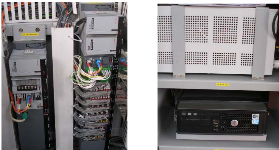
Figure 15. PLC (Programmable Logic Controller) & UPS
