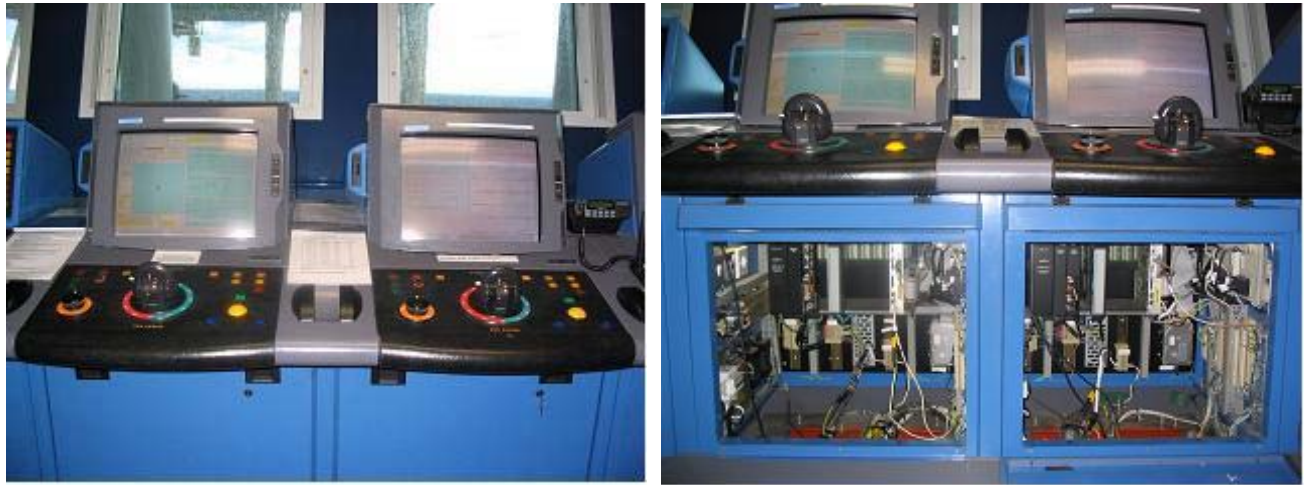
Figure 3 – pre-upgrade consoles and hardware
