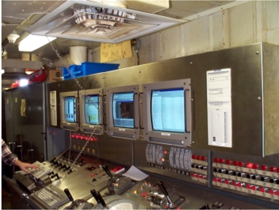
VMS Engine Control Room Console: Startup
